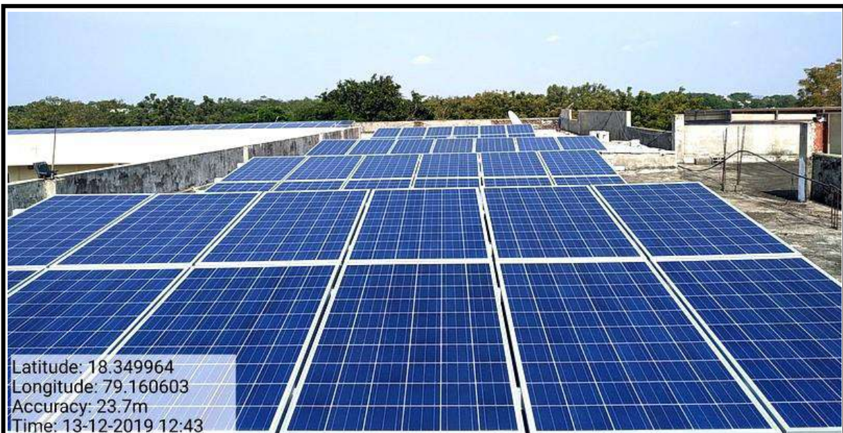
Solar Power Plant
